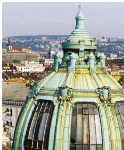
FIGURE 3.1.6 This copper roof has corroded to form a green coating called verdigris.
