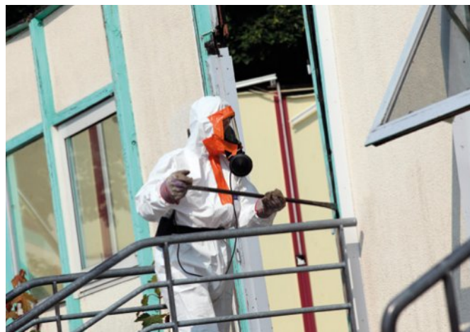
FIGURE 8.3.14 Workers removing asbestos from buildings must wear safety clothing and a mask.
