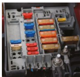
FIGURE 6.3.9 Each colour fuse in this car will melt at a different temperature and current.
