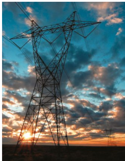
FIGURE 6.2.10 Transmission lines need to be made of a low-resistance, light metal. Copper would be far too heavy, so aluminium is used instead.
