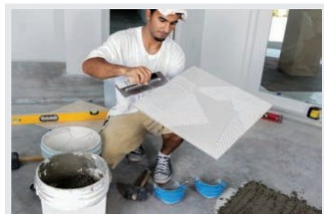
On a 20 kg bag of dry tiling adhesive the manufacturer's instructions might be to mix the 20 kg with 7.5 litres of water. A tiler can divide by the common factor 10 and simplify this rate to a more suitable rate of 750 mL water/2 kg of tile adhesive.
