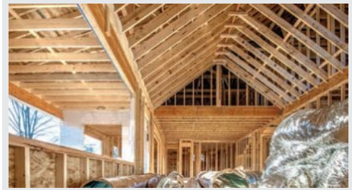
A builder makes sure that the roof rafters are all parallel, the ceiling joists are horizontal and parallel, and the wall studs are vertical and parallel.
