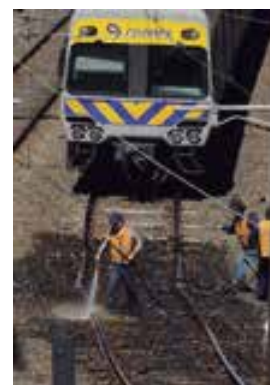
Figure 4.26 Train tracks would buckle in the heat without tiny gaps between them.
