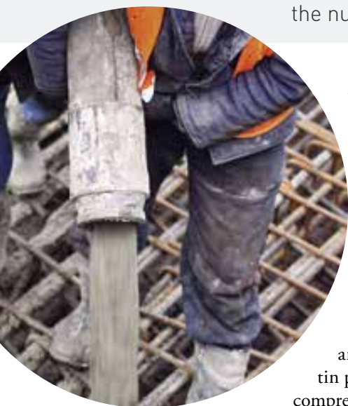
Figure 4.13 Reinforced concrete combines the tensile strength of steel with the compressional strength of concrete.
