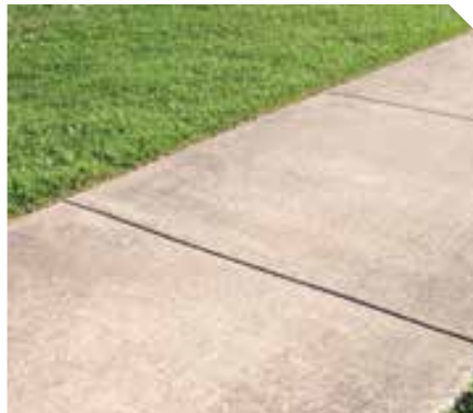
Figure 2.41 Temperature erosion causes materials such as concrete to crack. Footpaths have grooves in them to allow for their expansion during hot weather.
